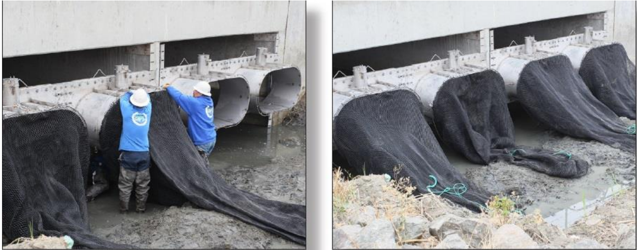
Figure 2 - Example of a Trash Capture Device Under Consideration - Oldcastle Stormwater Solutions NetTech Gross Pollutant Trap, City of Vallejo.
