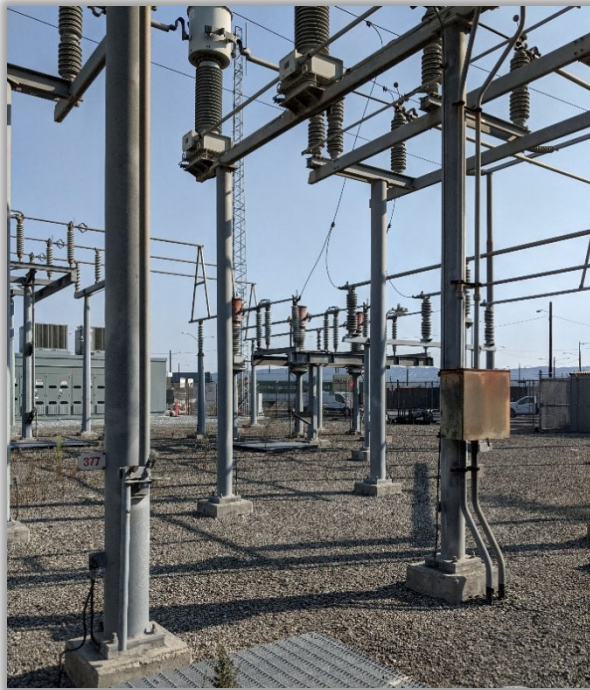
Port of Oakland Electrical Substation
