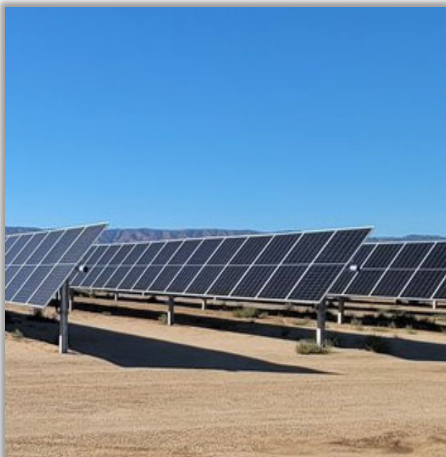
Port Utility solar array
