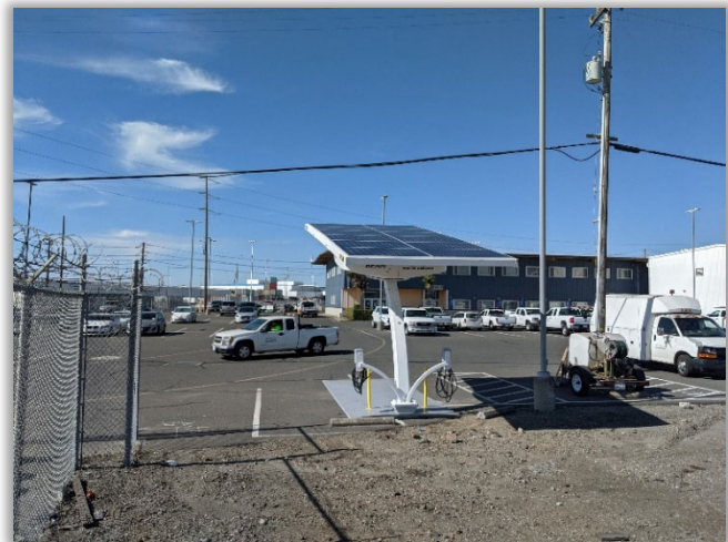
Electric Vehicle Charger at Port's Harbor Facilities Complex
