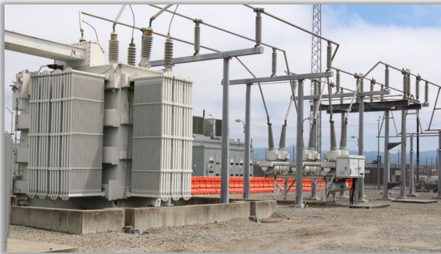
Port of Oakland Davis / Cuthbertson Electrical Substation
