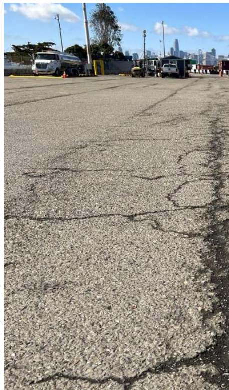
Figure 1 AC Condition Example
