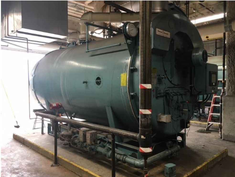
Figure 1 – Existing Terminal 2 Natural Gas Fired Boiler.
